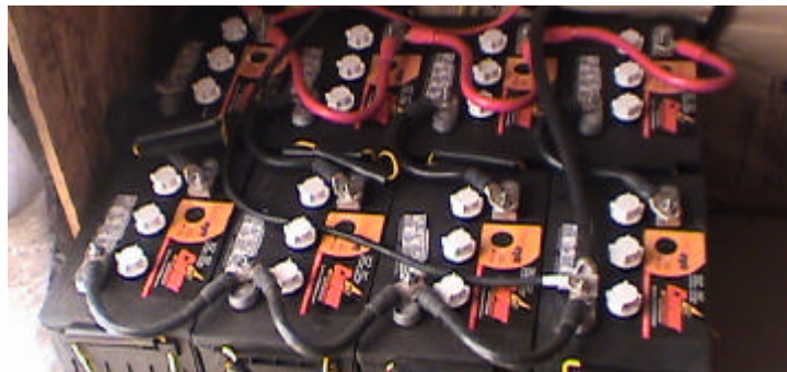
Typical residential battery bank.
