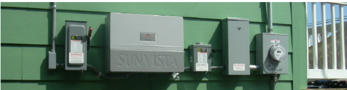
Pictured from left to right are the following solar electric system components of a grid tie system. 1) solar array manual disconnect (code required), 2) inverter, 3) A/C manual disconnect (required by net metering regulations), 4) distribution panel and 5) utility meter.
