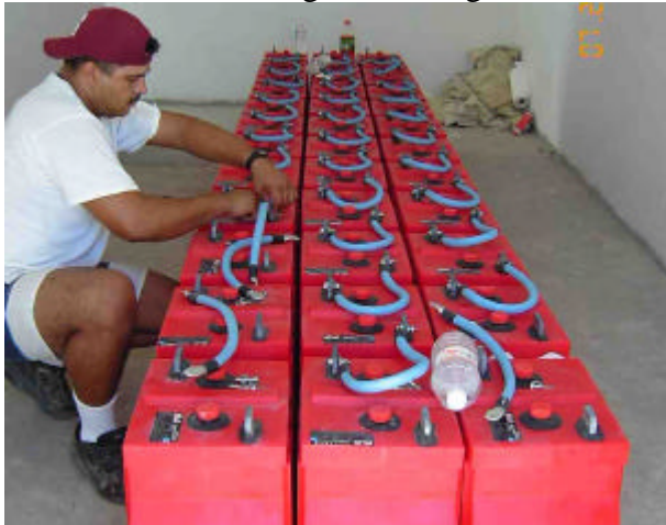
Typical small commercial battery bank.
