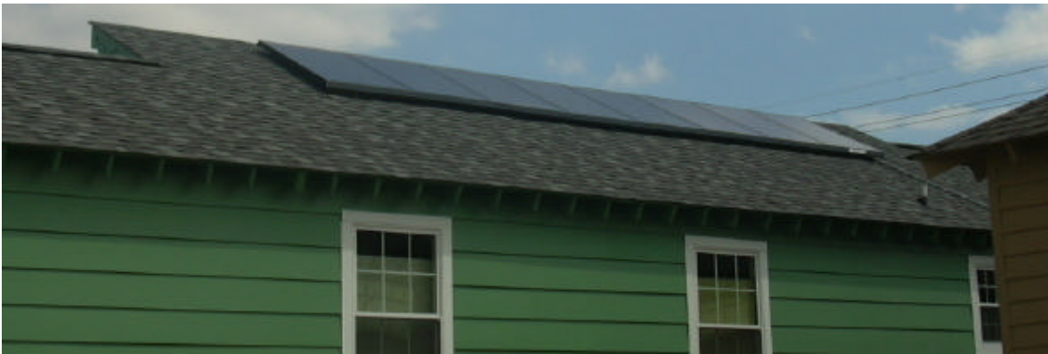
Pictured above is one of the 10 net metering solar energy systems recently installed in the Ninth Ward in New Orleans by Sharp Solar. The 1.5 KW (1,500 watt) solar array is composed of eight separate solar panels.
